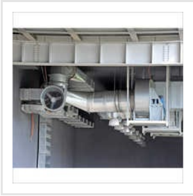
GI Ducting System
